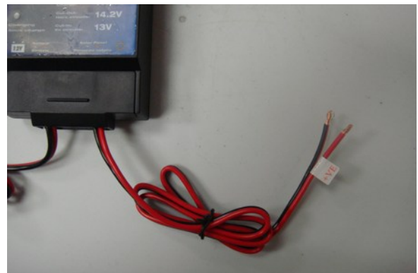
Figure 3: Solar Panel Array wires lead from Charge Controller
