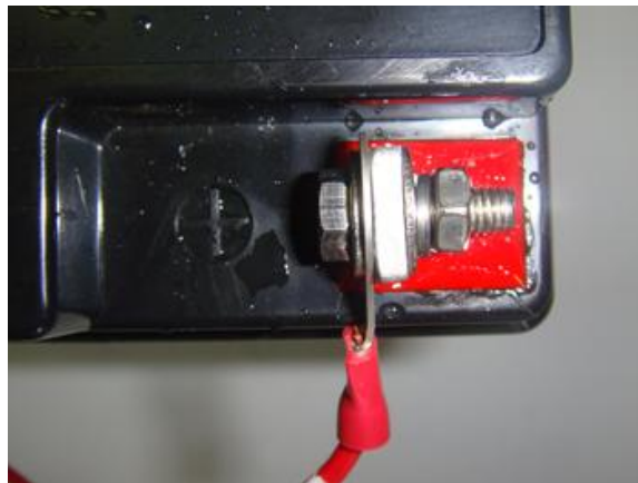
Figure 2: Bolt, washers and nut used to connect wire terminal to positive battery terminal (red with + sign)
