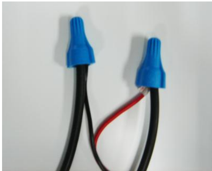
Figure 6: Connected Solar Panel and Charge Controller Wires
