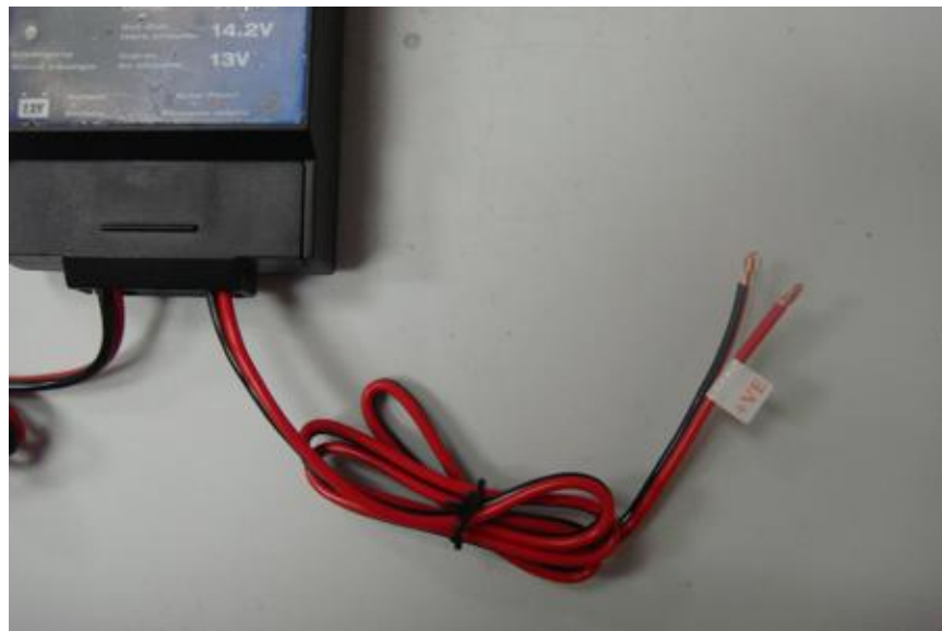
Figure 4: Solar Panel Array wires from Charge Controller
