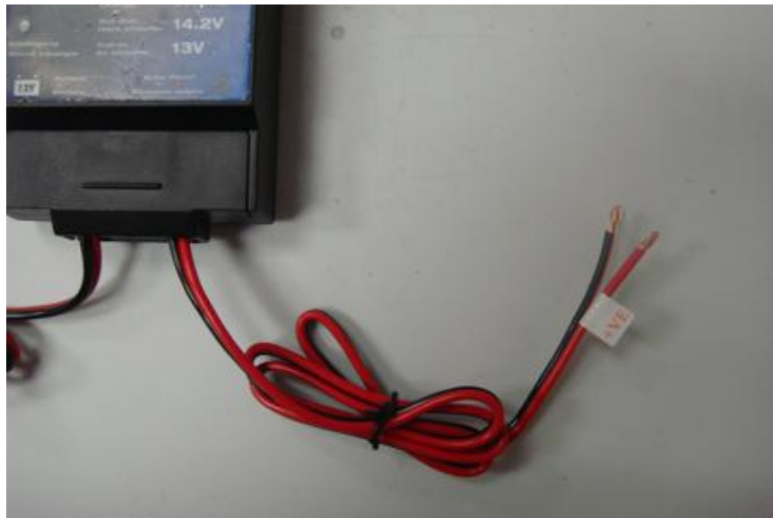
Figure 4: Solar Panel Array wires from Charge Controller
