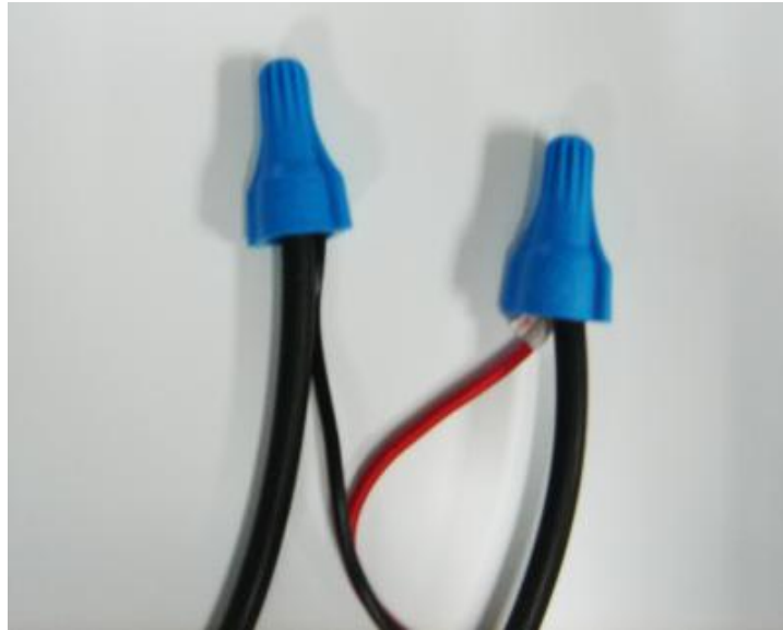
Figure 5: Connected Solar Panel and Charge Controller Wires
